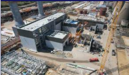
Mintia Power Plant 1.750MW (Romania)
